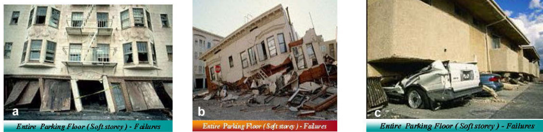
Fig. 2. Damages of structures with stilt structure: Left (a), three storey, center (b) two storey, and right (c), damage to a parking lot.
